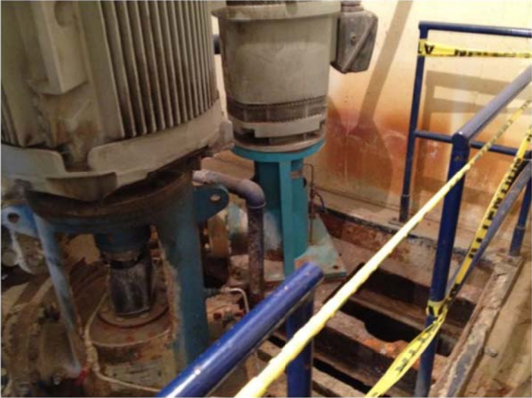
West Kelowna Estates Intake Pump Station
