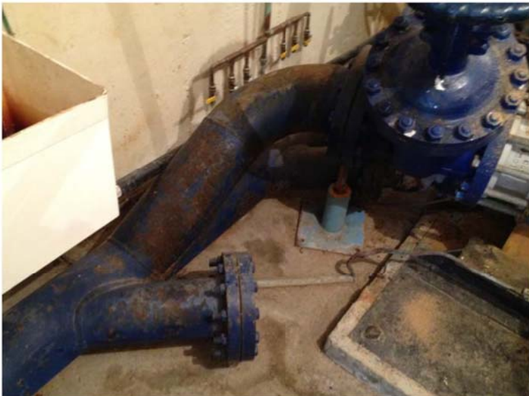
West Kelowna Estates Intake Pump Station
