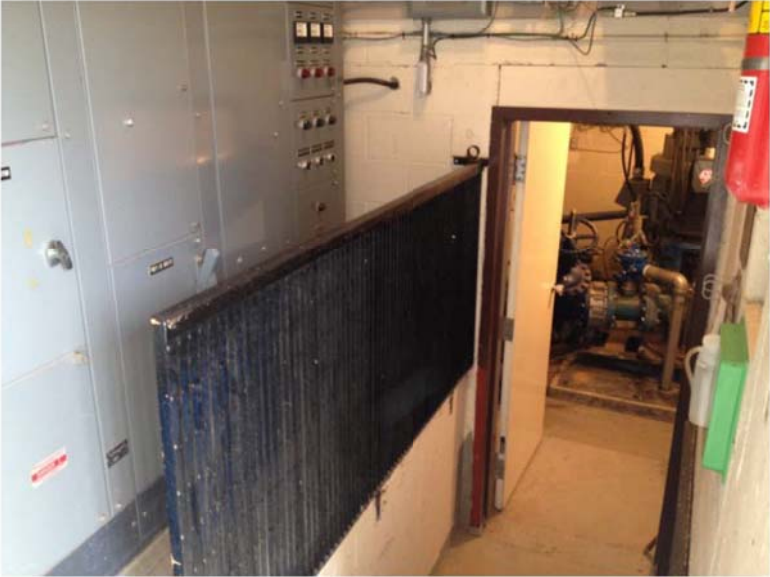
West Kelowna Estates Intake Pump Station
