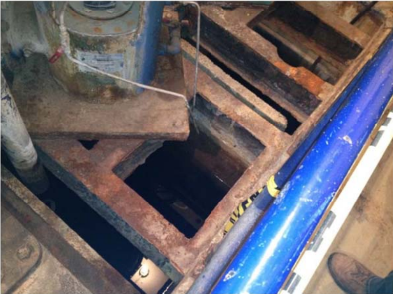
West Kelowna Estates Intake Pump Station
