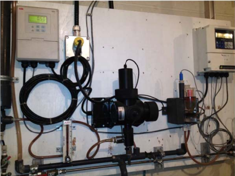
West Kelowna Estates Intake Pump Station
