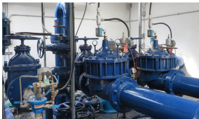
Figure 17: Pump Station Interior
