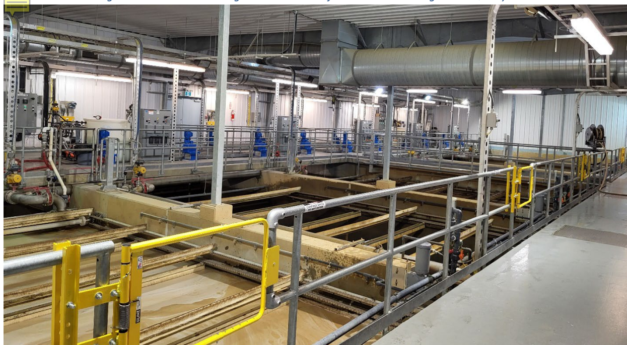
Figure 8: Inside the Powers Creek Water Treatment Plant
