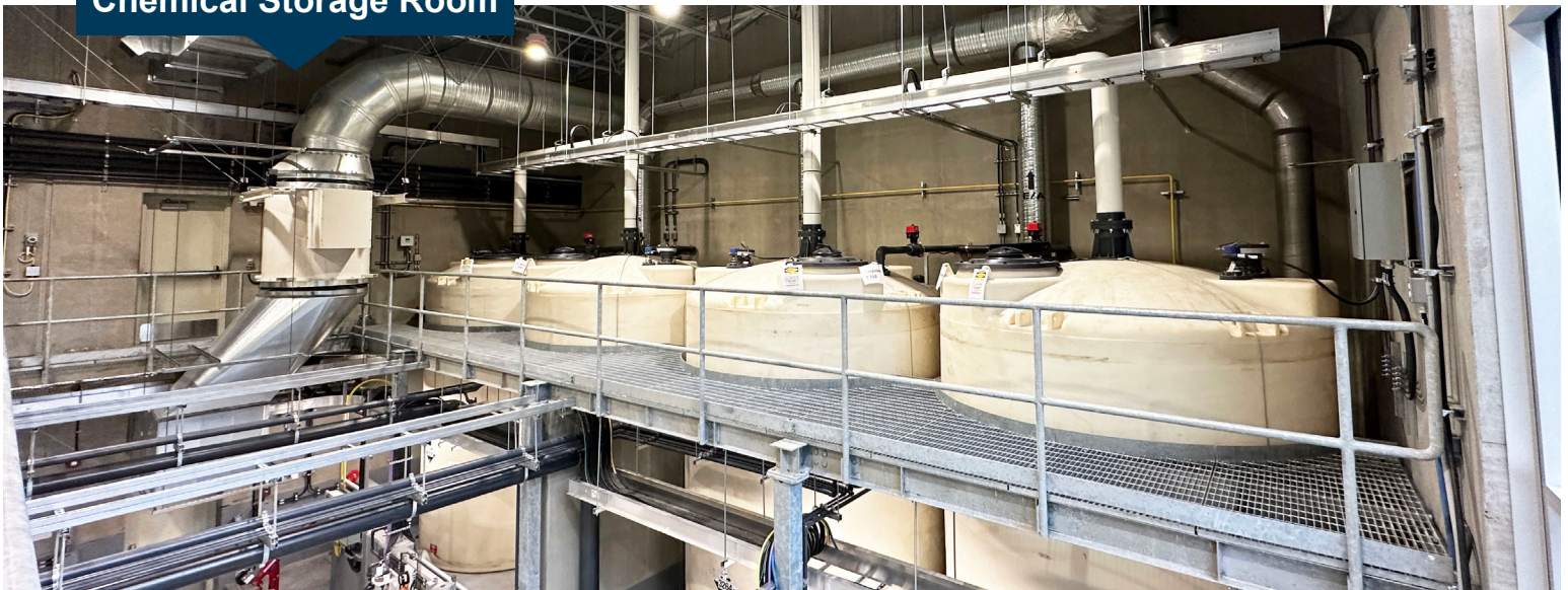
Chemical Storage Room
