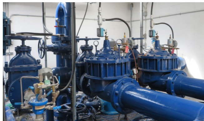
Figure 16: Pump Station Interior
