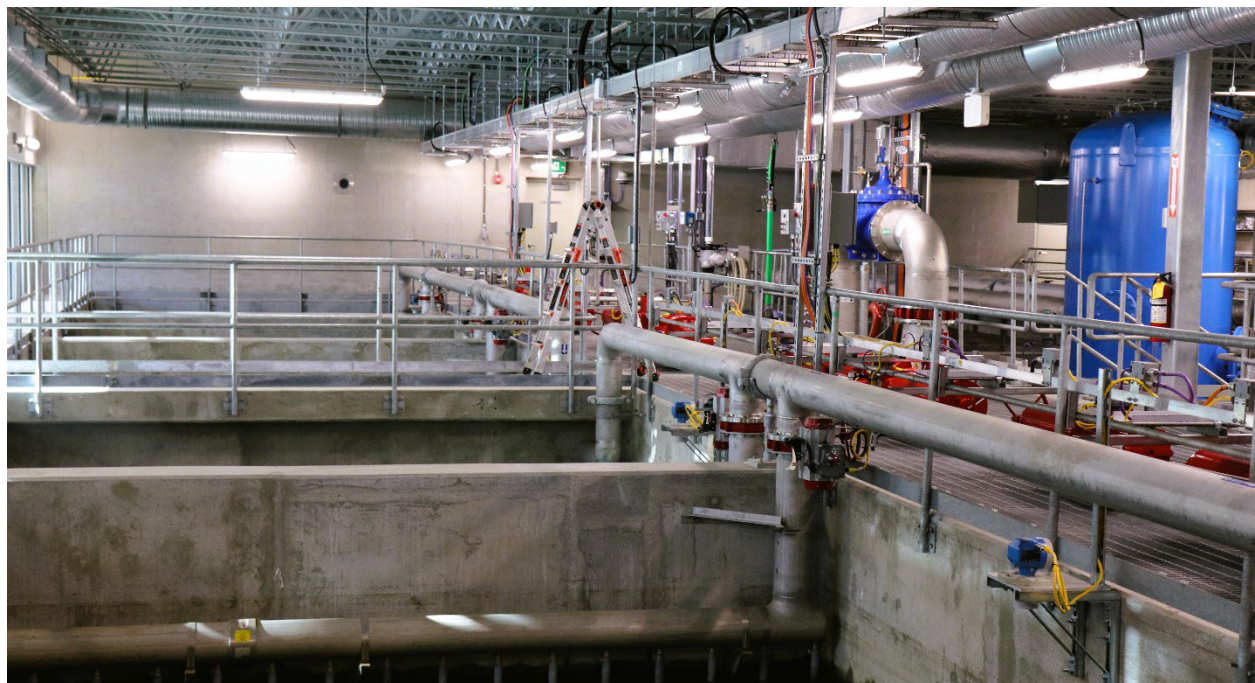
Figure 8: Inside the Rose Valley Water Treatment Plant
