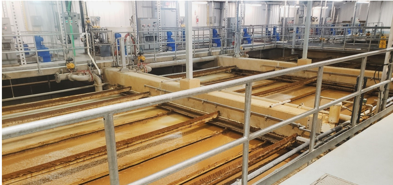
Inside view of Powers Creek Water Treatment Plant
